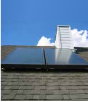
Vitosol 200-F flat plate solar collectors.
