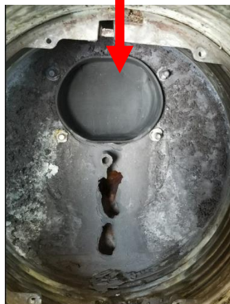
Accelerated corrosion on aluminum back plate of heat exchanger
