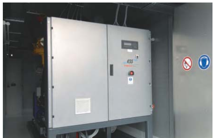
The CHP unit meets four percent of electrical demand and three percent of thermal needs at the Allendorf facility.
