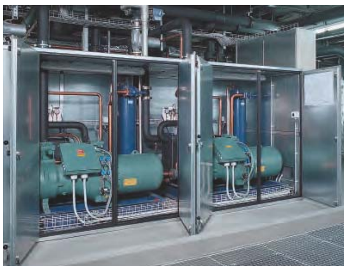
KWT ground source heat pump with heating output of 500 kW at Berna Biotech AG, a vaccine producer in Bern, Switzerland.
