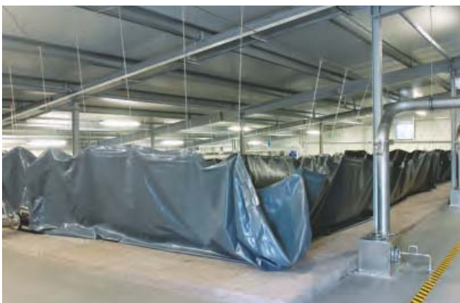
Gas bags serve as intermediate storage for biogas.
