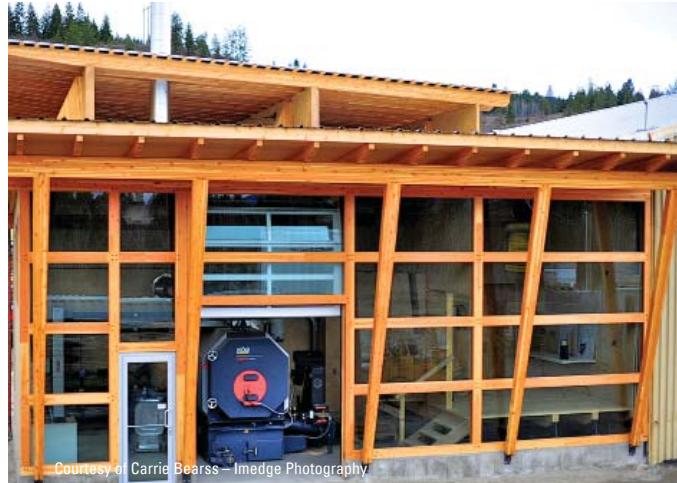
Custom-built boiler house with wood chip fuel storage bunker and walking floor feed system
