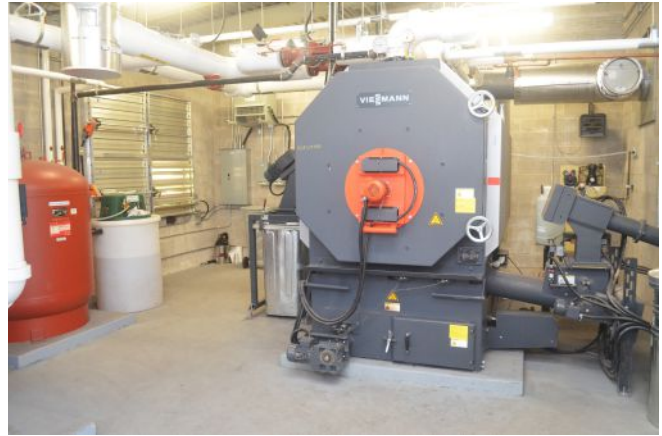
Instead of purchasing new oil-fired units, two high schools in New Brunswick replaced a significant portion of their fossil fuel load with biomass-fuelled boiler systems.
