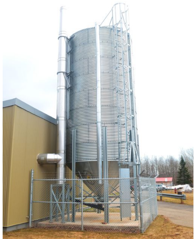
The biomass boiler system at Sussex Regional High School includes a 60-ton wood pellet silo.
