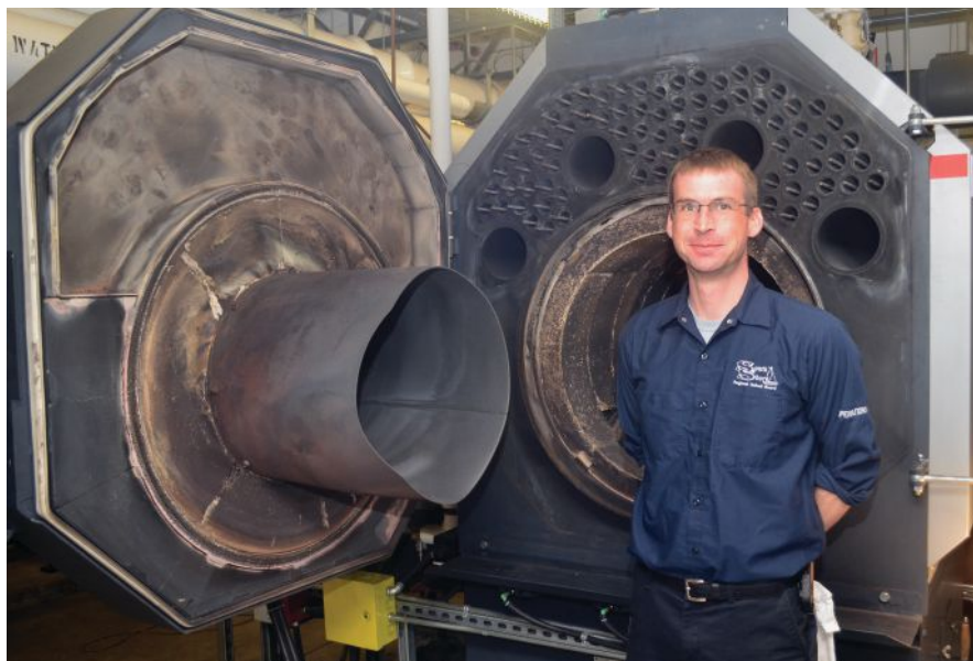
Adam George is responsible for the maintenance of Bluenose Academy's biomass heating system, in addition to other biomass hot water boilers installed at schools across the South Shore Regional School Board in Nova Scotia.
