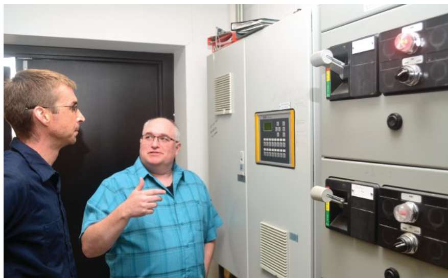
The entire system is controlled by a Viessmann master control that communicates via a local operating network control module to all the boilers and runs them when needed.
