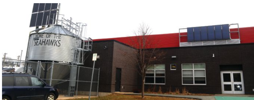
A Viessmann Pyrot 540kW wood pellet-fuelled biomass hot water boiler is the school’s primary source of heat for fuelling the school’s hydronic heating system.
