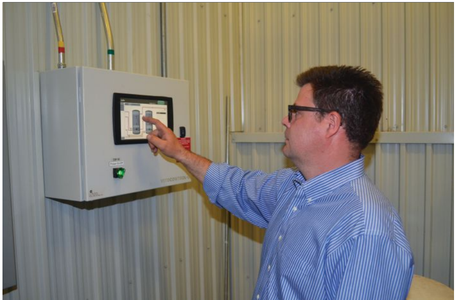
Daron Thomas of Thomas Industrial Sales checks out the master control panel for the new radiant heating system at Les Residences Jodin.
