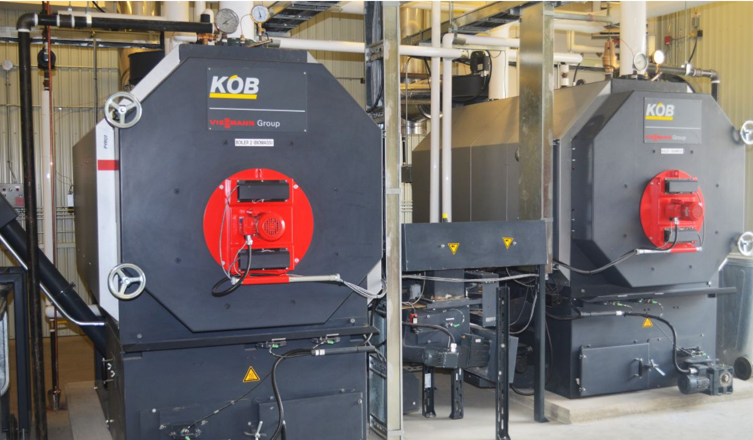
Two Viessmann biomass boilers were installed to produce the primary heat for the radiant heating system at Les Residences Jodin, a nursing home in Edmundston, N.B.
