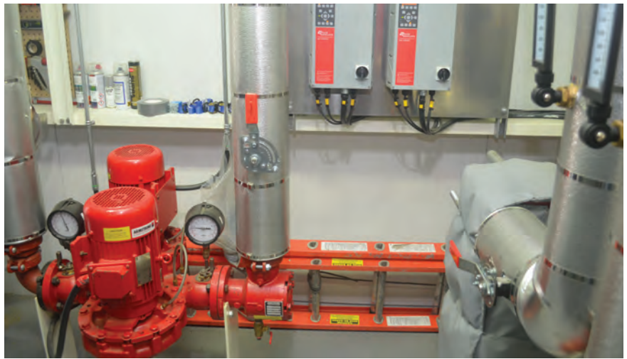
The hot water from the buffer tank is pumped via two Armstrong variable speed pumps at a flow rate up to 120 USgpm into the distribution system in the building’s mechanical system.
