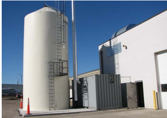
A containerized system with Pyrot KRT-150 boiler, peripheral equipment and wood chip silo simplified the heating system retrofit
