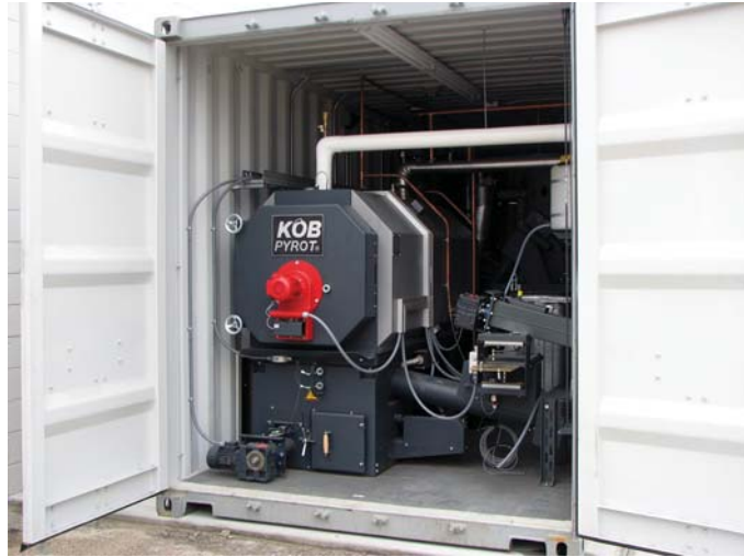
A Viessmann Pyrot KRT-150 boiler utilizes locally-sourced wood biomass fuel to heat the 2,365-square-metre Camrose County Administration Office
