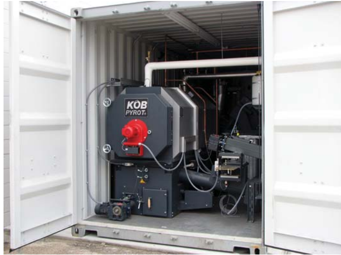
A Viessmann Pyrot KRT-150 boiler utilizes locally-sourced wood biomass fuel to heat the 2,365-square-metre Camrose County Administration Office
