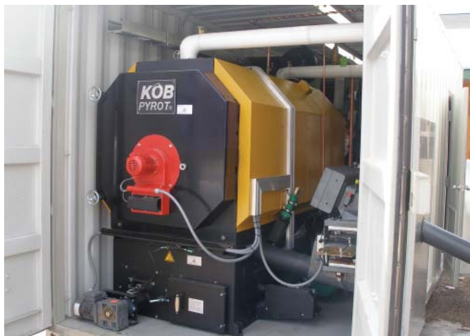
A containerized system with Pyrot KRT-300 boiler, peripheral equipment and pellet silo simplified the two-day installation process
