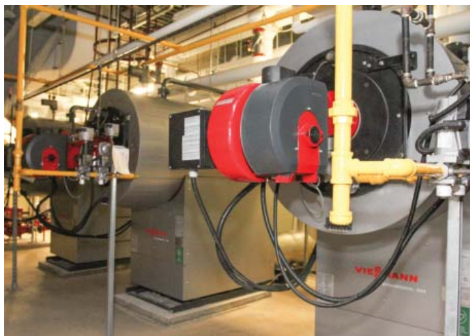
Three Vitocrossal 300, CT3 boilers provide heating for the viewing gallery and ice and snow melt system
