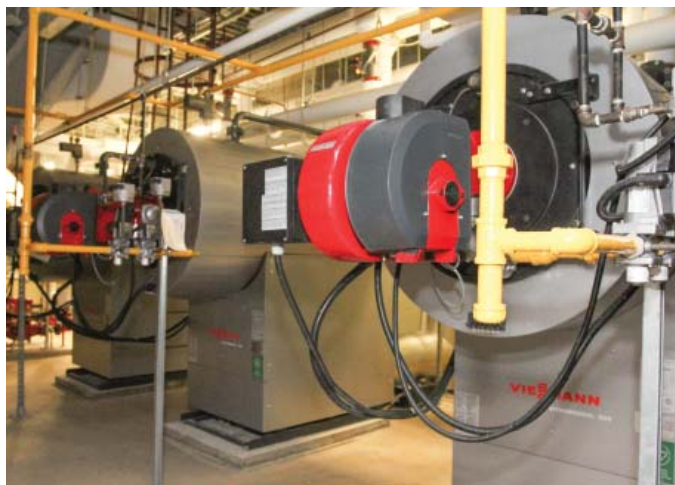
Three Vitocrossal 300, CT3 boilers provide heating for the viewing gallery and ice and snow melt system
