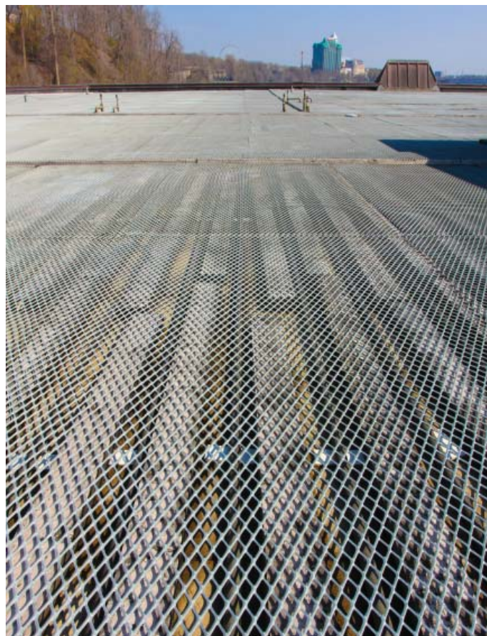
Wood racking and metal mesh offer protection for the rooftop ice and snow melt system's copper piping
