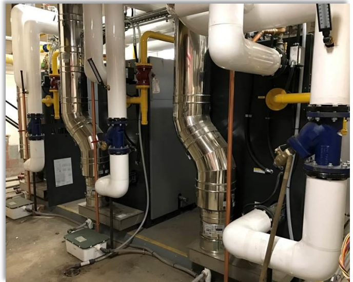
Viessmann Vitocrossal 300, CA3 condensing boilers (4000 MBH)*
